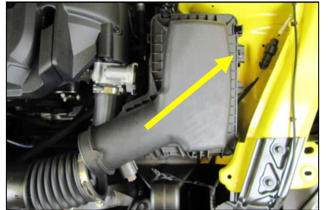
3. Remove the 6mm airbox mounting bolt in the inner fender and lift the entire airbox assembly out of the vehicle. Set the bolt aside for now. It is to be reused.
